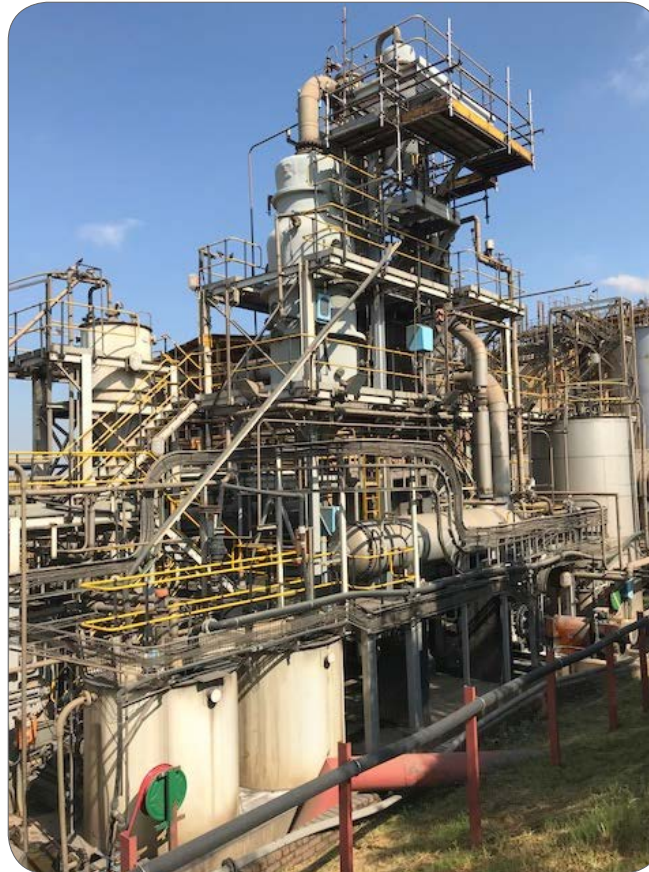
Second stage evaporator
