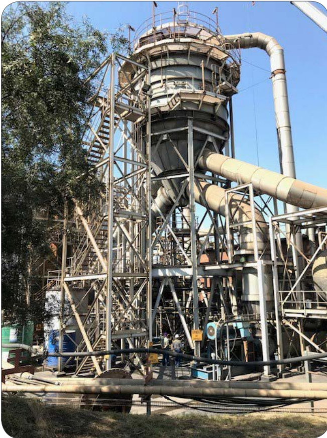
Second stage evaporator
