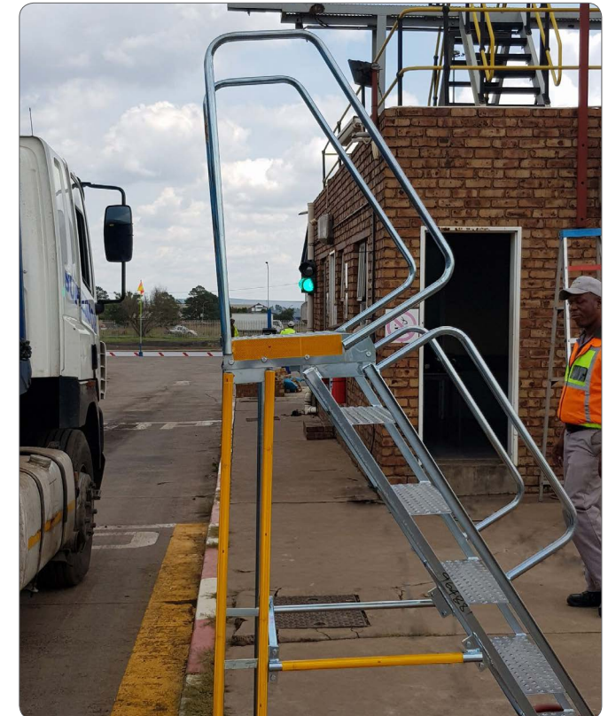
Ladder in home position, green light will be visible (cables re-routed to minimise tripping hazard)
