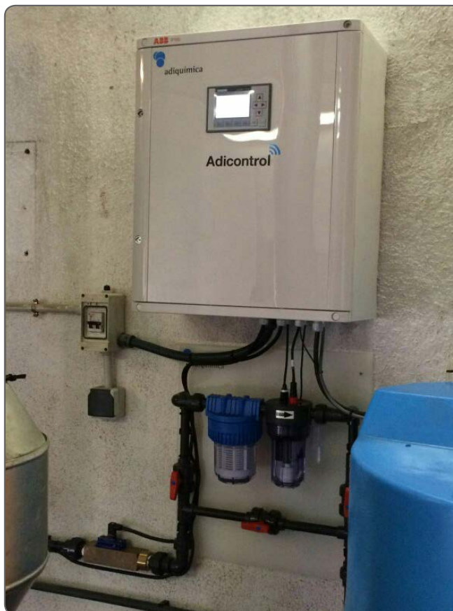
Detail of control panel
